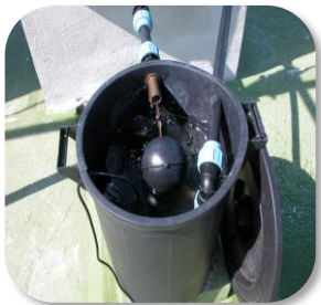
External tank and pump with float
